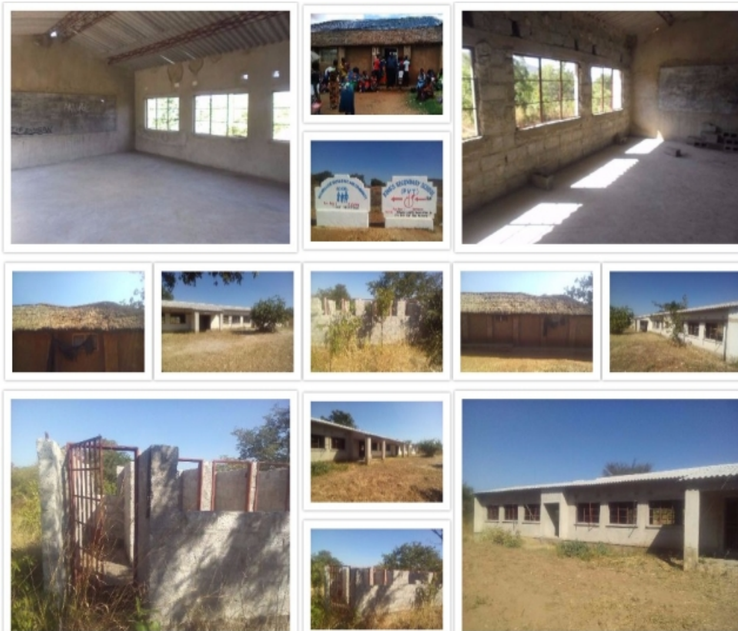
clinic that needs new roof and the high that needs completions together with ablution blocks
